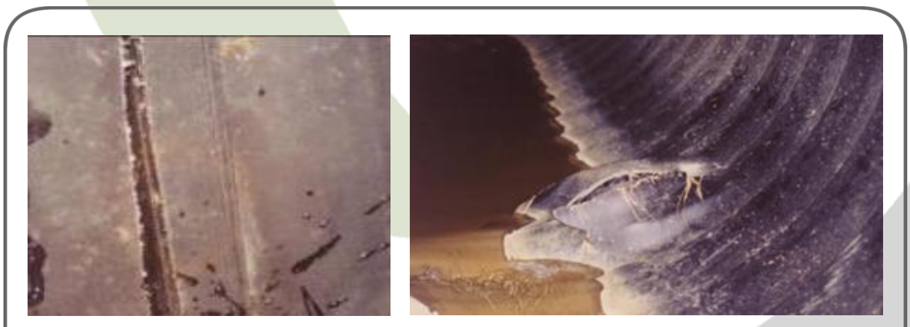
Figure 5. Cases of plastic pipe bulges and cracks from the survey (2002)
