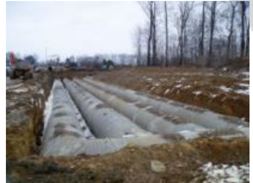
Detention system to accommodate 4 equal runs of pipes, 8 fabricated fittings and no short joints
