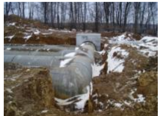
Tees & bends to form manifold of structure
